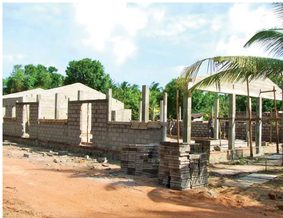
The new brick church being built by Pastor Gnanasundaram. His first wooden church was burned down – twice.
